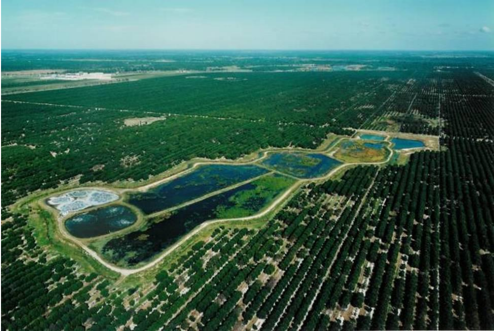
This is a treatment system for a large citrus processing plant in Florida
